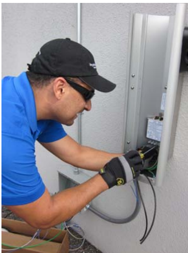
Gabriel Regalado of Regalado Electric wires an EVSE at Zero Motor Cycles in Scotts Valley.
