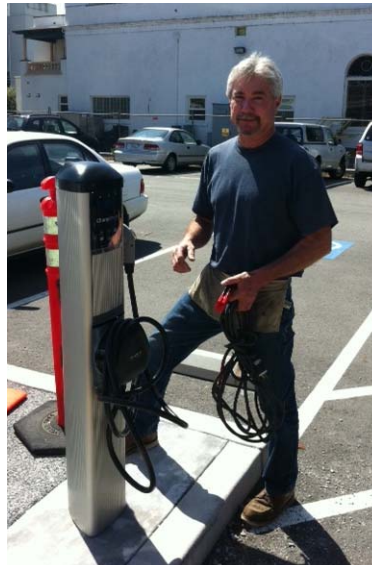
Brett Ritchie of Central Electric finishes an EVSE installation at Ecology Action in Santa Cruz
